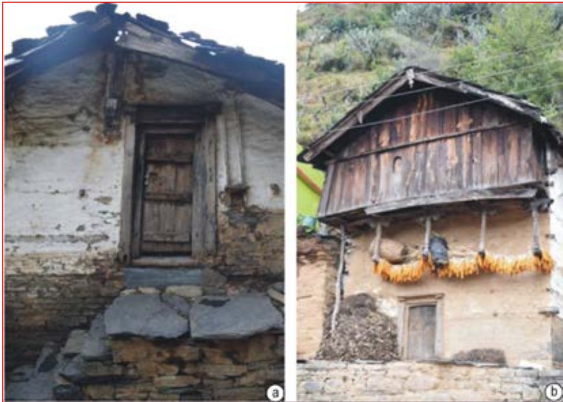
Fig. 12. (a-b): More than 100-year-old houses.
